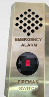
EMERGENCY ALARM CUM FIRE MAN SWITCH
